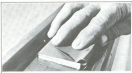
Figure 2J-6. Sanding Patch
